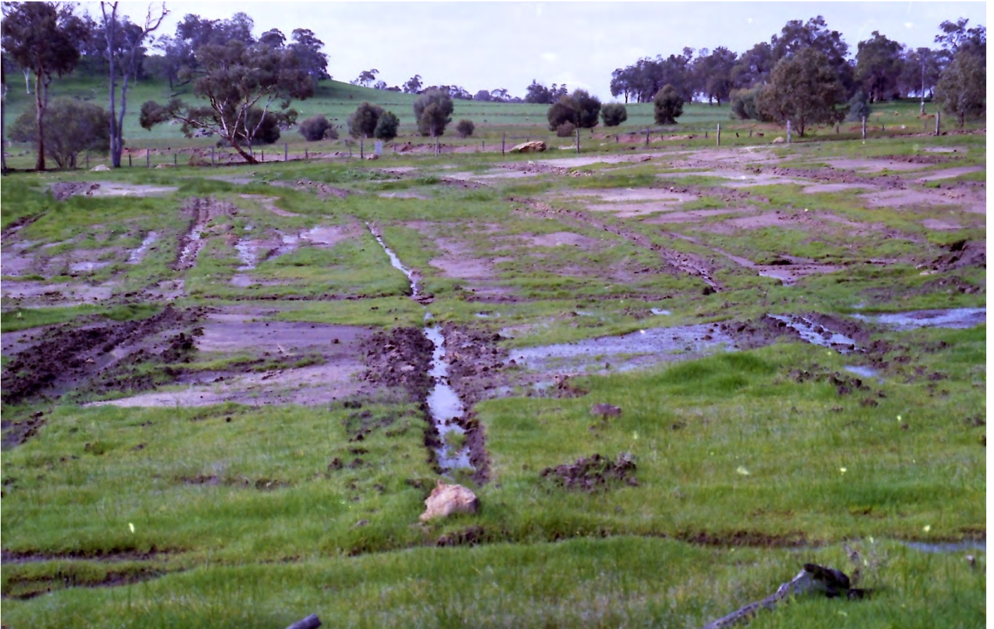
Above: Ground water seepage at the Laurie Chitty Project on Toodyay Road, 26th March 1991
